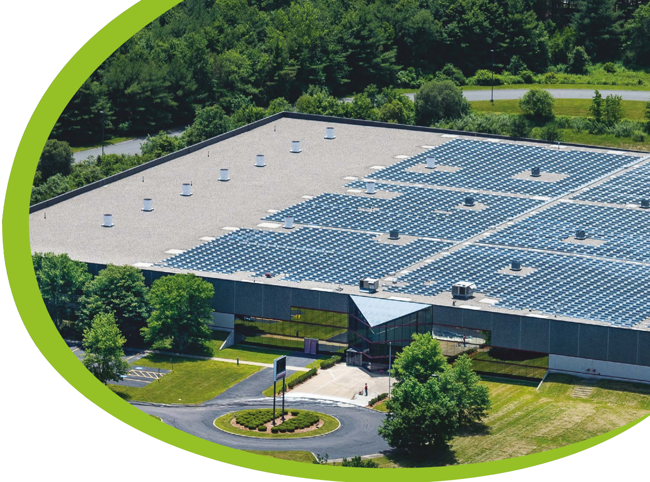
SED Solar Portfolio - rooftop solar system installed at an industrial facility in Massachusetts
