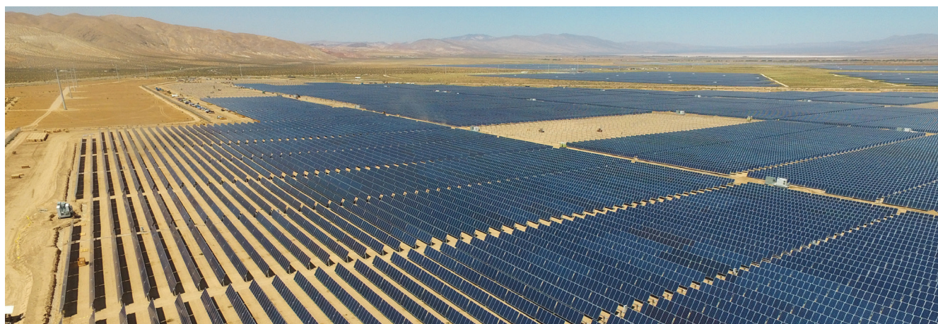
Beacon 5 – ground mounted solar project in California
