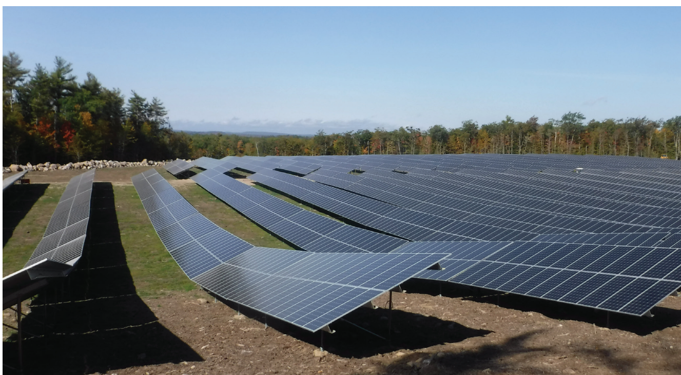
Ellis Road Solar in Massachusetts
