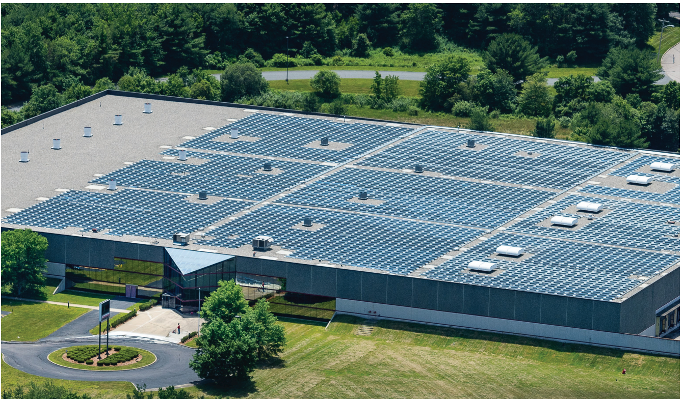
SED Solar Portfolio – rooftop solar system installed in Massachusetts
